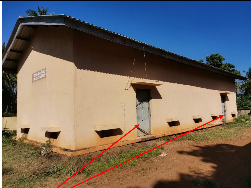
Existing Doors of the fertilizer store - small space for entrance, the space not enough for vehicular movement and fertilizer transport.
